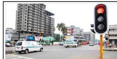
Figure 1.62 - Traffic Lights Control System
